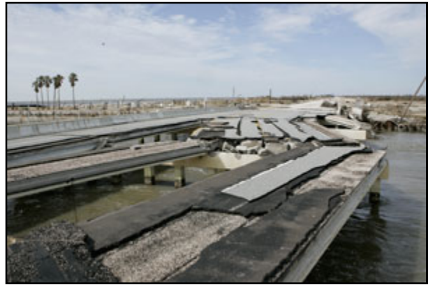
Figure 29. Damage to SH 87 at Rollover Pass Bridge, Bolivar Peninsula
