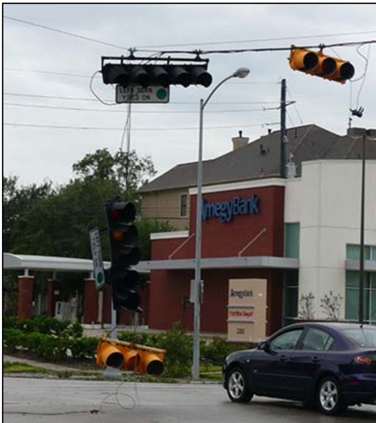
Figure 31. Traffic Signal Damage, City of Houston (ABC News)
